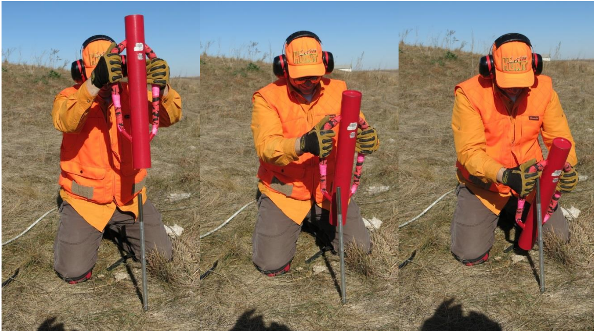
Figure 15. Demonstration of a dangerous method using the post driver. If the post driver is raised above the rod during the upward swing (first picture), it can miss the rod (second picture), and injure the worker’s hand or leg (third picture).
