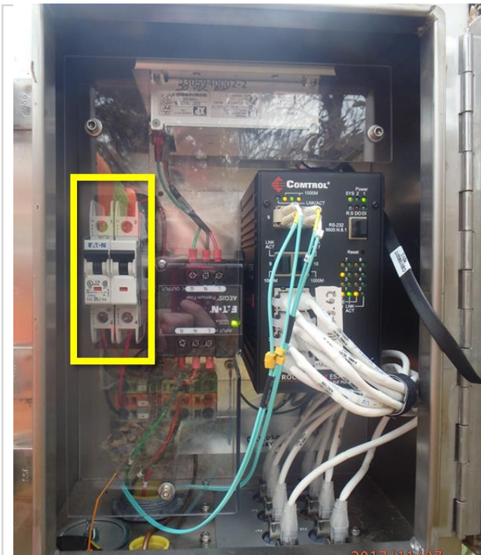
Figure 123. AIS Combination Box - 5 Amp Breakers
