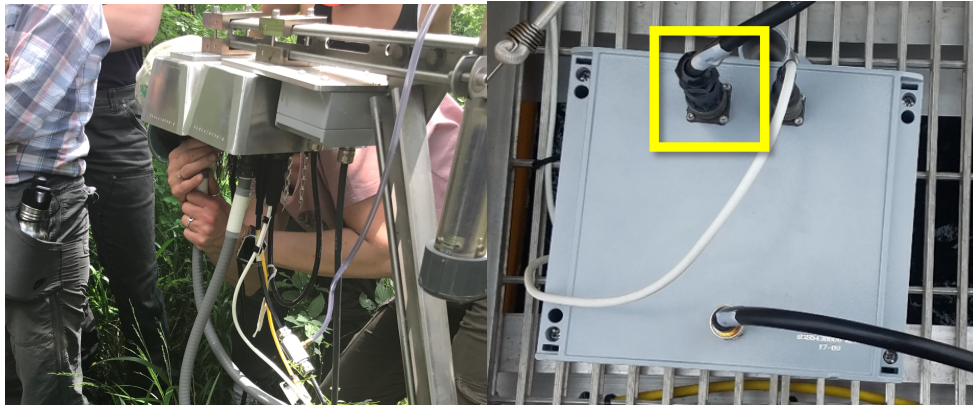
Figure 11. Disconnect the SUNA power source for wadeable streams (left) and buoys (right).
