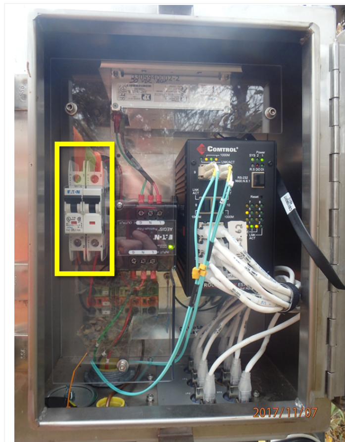
Figure 58. AIS Combination Box - 5 Amp Breakers.
