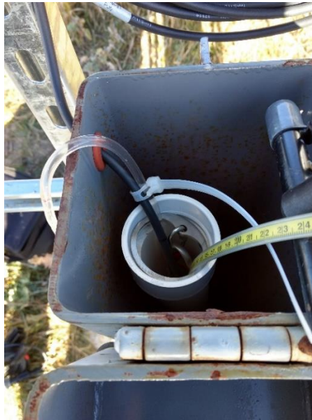
Figure 28. Pump tubing secured in place with zip tie.
