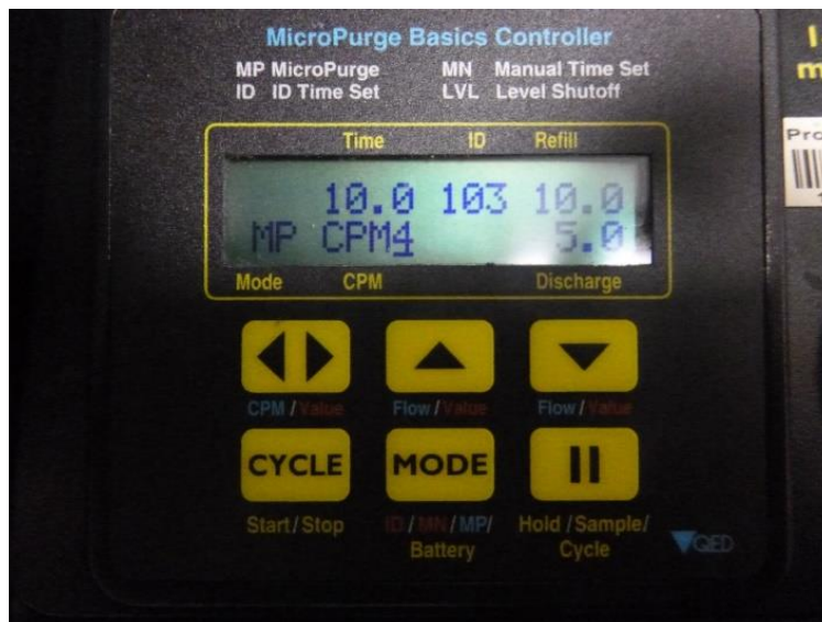
Figure 26. Groundwater pump control panel screen. Note the Refill and Discharge times on the right.
