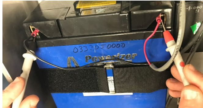
Figure 48. Use a DMM to Verify Battery Voltage
