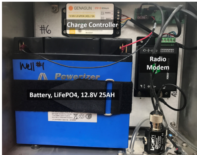
Figure 5. Power/Telemetry Components in GWW NEMA Enclosure
