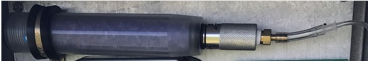
Figure 27. Desiccant in Radio Box with Vent Tube Attachment Close-up
