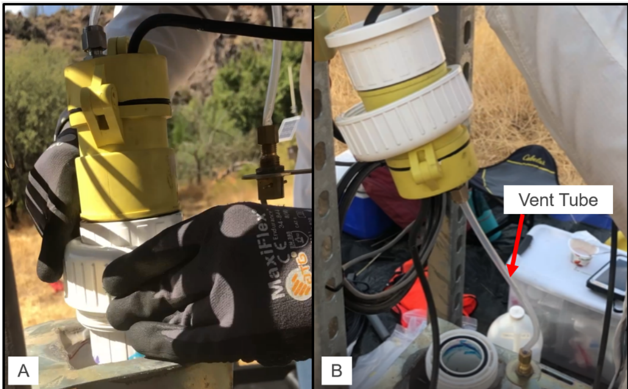
Figure 10. A) Snorkel Cap Modification for Flood-Risk Sites & B) Vent Tube with Snorkel Cap Removed
