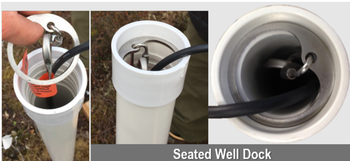
Figure 69. Well Dock in PVC casing
