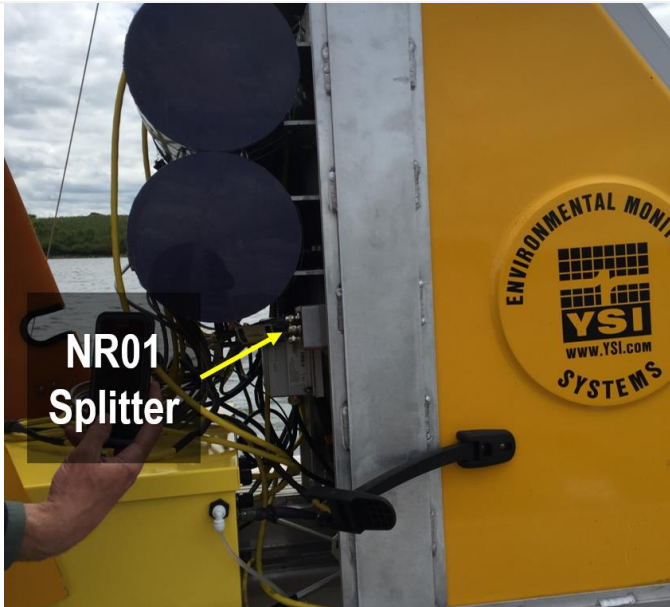
Figure 103. Net Radiometer Splitter on AIS Buoy on T-Frame
