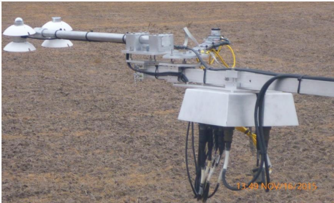
Figure 56. Tower Top ML Combined Boom Radiation Sensor Subsystem Grapes (D06 KONA)
