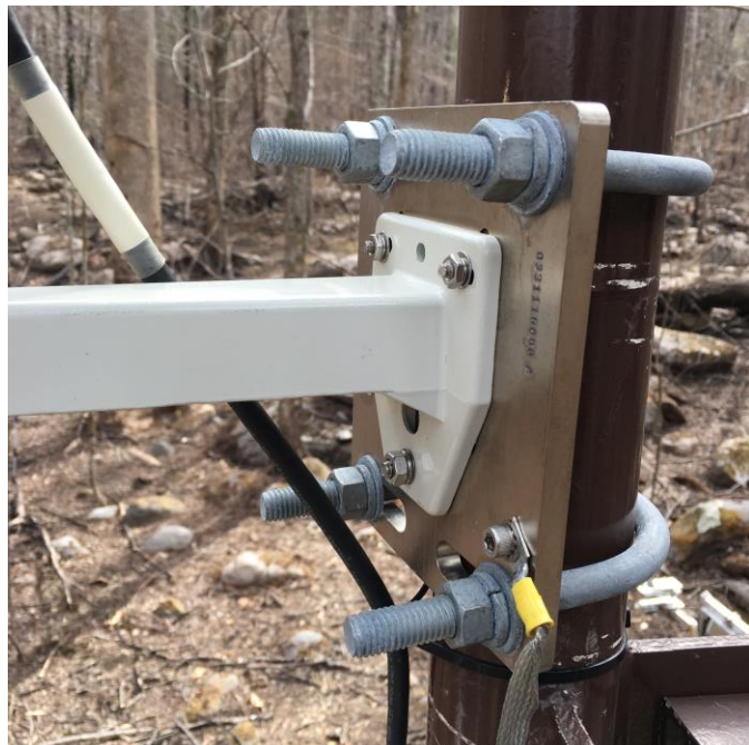
Figure 13. Camera U-bolts and Grounding Cable on TIS Tower Leg
