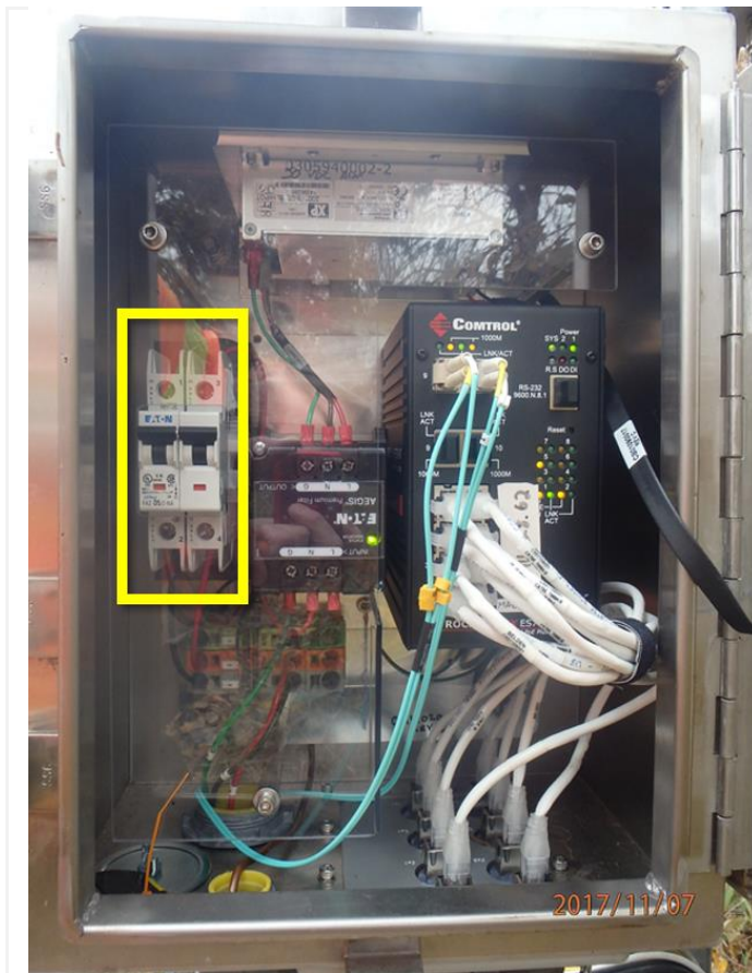
Figure 68. AIS Combination Box - 5 Amp Breakers
