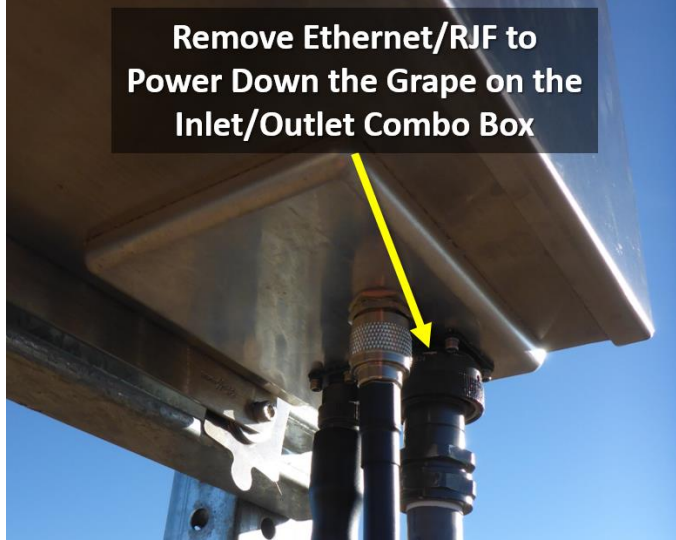
Figure 12. Power Down Site from Combo Box
