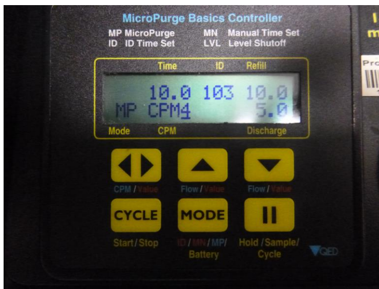
Figure 20. Groundwater pump control panel screen. Note the Refill and Discharge times on the right.
