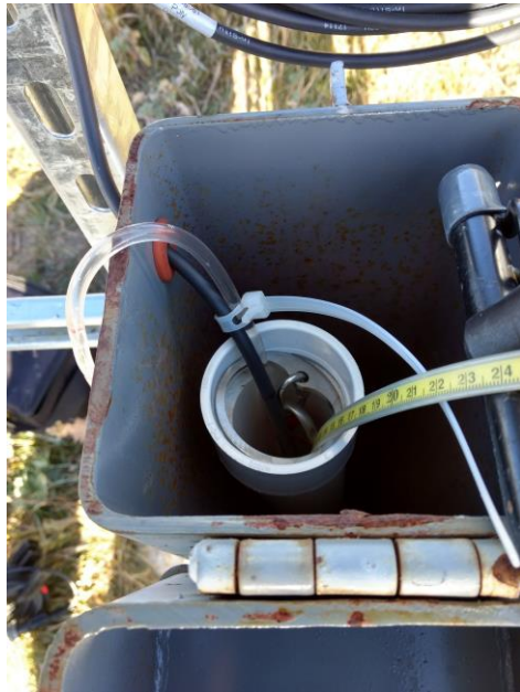
Figure 21. Pump tubing secured in place with zip tie.
