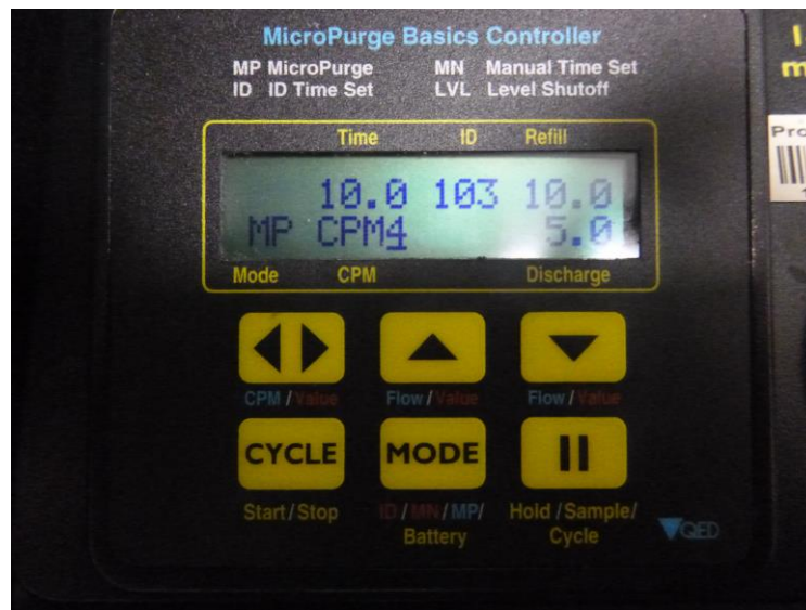
Figure 20. Groundwater pump control panel screen. Note the Refill and Discharge times on the right.
