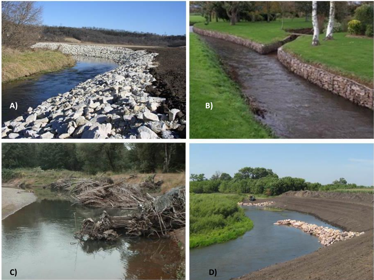
Figure 12. Examples of shoreline revetments a) rip-rap with rock, b) gabion baskets filled with rock, c) soft armoring using root wads and logs, and d) in-stream rock J-hook for modifying flow.
