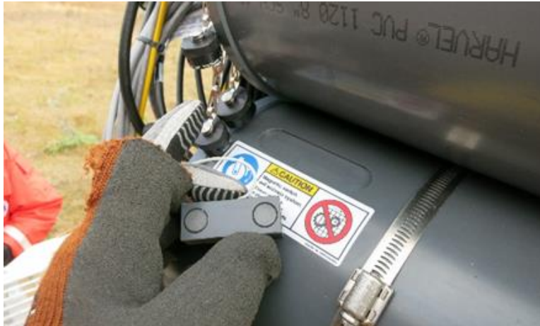
Figure 36. Magnetic Switch to Activate the Winch
