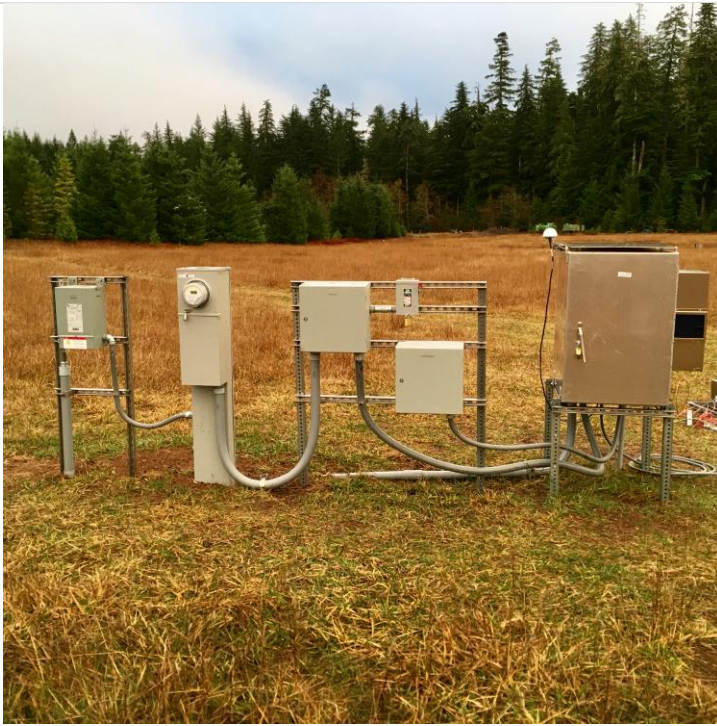
Figure 13. Associated infrastructure for the Primary Precipitation Gauge.
