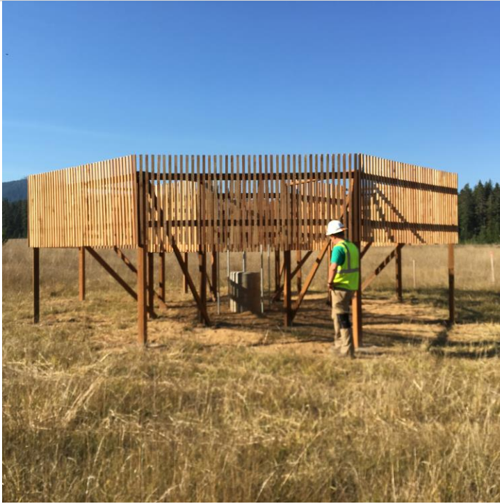
Figure 3. Side view of a NEON DFIR. This displays a non-standard (i.e. taller) DFIR fence heights (see Appendix 8.6.4).
