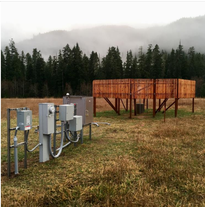
Figure 12. View of the DFIR fences and associated infrastructure.
