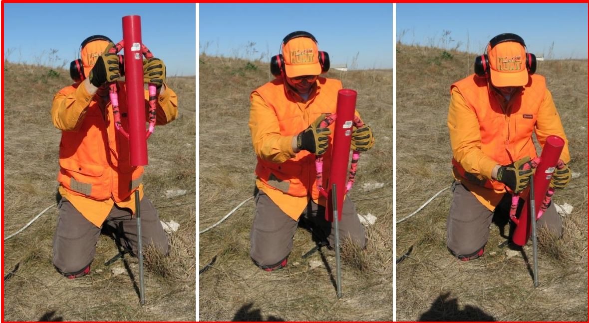
Figure 19. Do not lift the post driver above the top of the rod during the striking motion as the worker could injure their leg or hand
