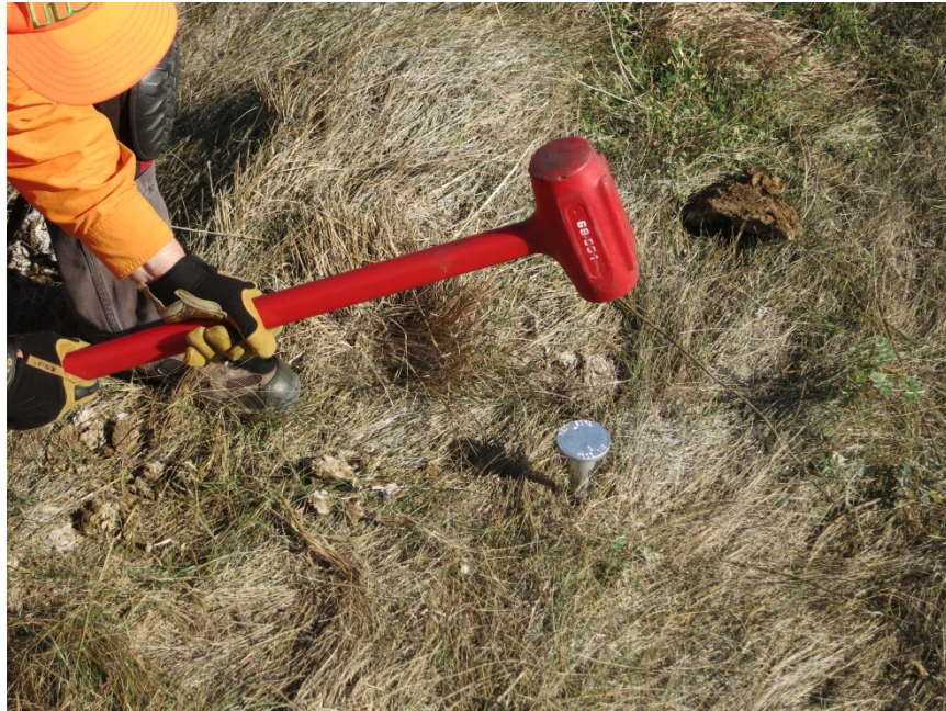
Figure 15. Use a sledgehammer to seat the cap and drive the rod to the desired position.
