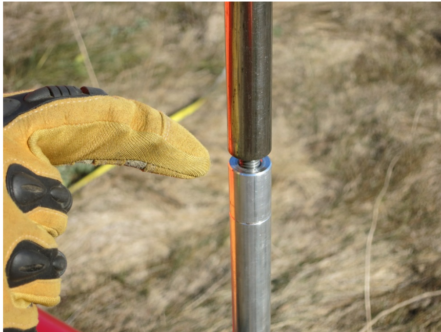
Figure 13. Picture of rod assembly sections separating while driving the monument, be sure to tighten before continuing.
