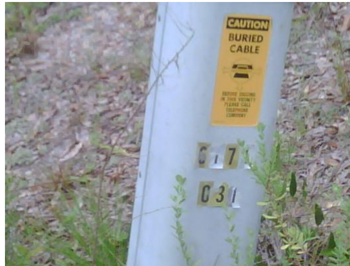
Figure 13 The power pedestal nearest Barco Lake.
