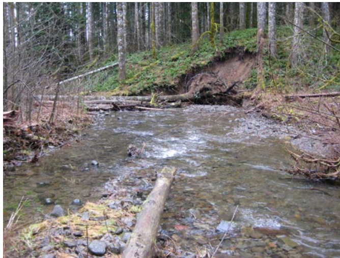
Figure 12 Occasionally, no riparian floodplain is present where a steep slope abuts against the channel in Martha Creek and shows signs of erosion. Shown here is the right bank between S1 and S2.
