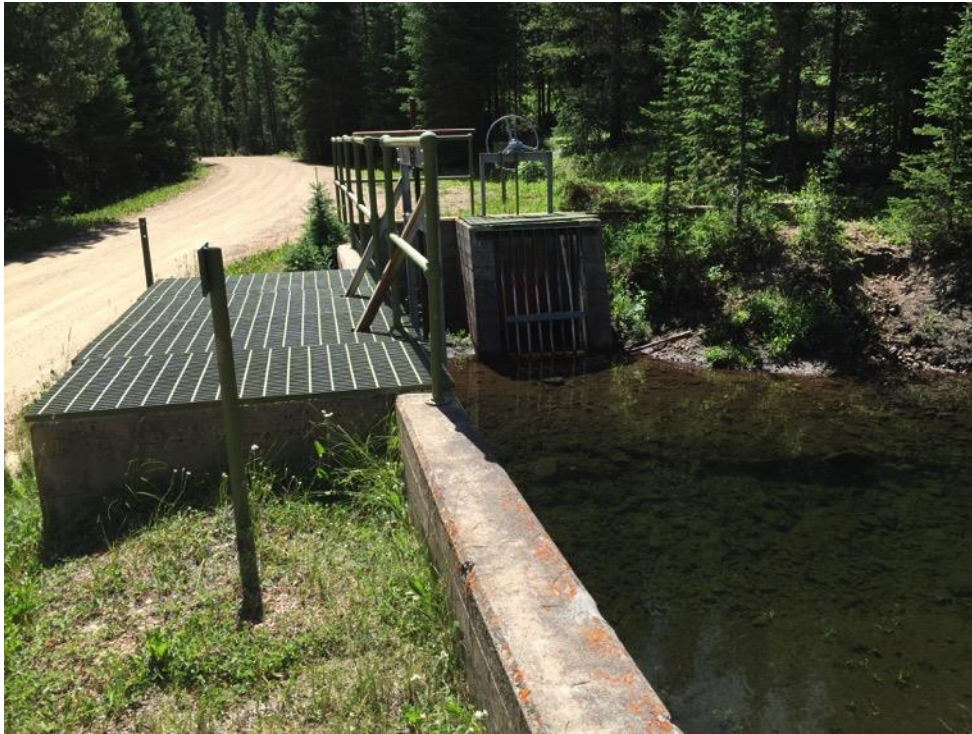
Figure 39. Picture of water diversion system installed on West St. Louis Creek downstream of the AQU reach at the access road.
