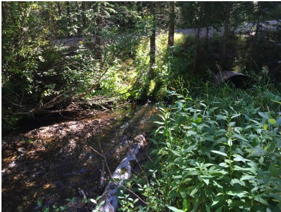
Figure 48. Picture of pool on upstream side of culvert where AQU reach passes the road to Byers Peak Trailhead.
