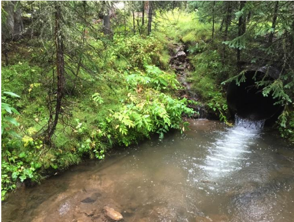
Figure 47. Picture of pool on downstream side of culvert where AQU reach passes the road to Byers Peak Trailhead.
