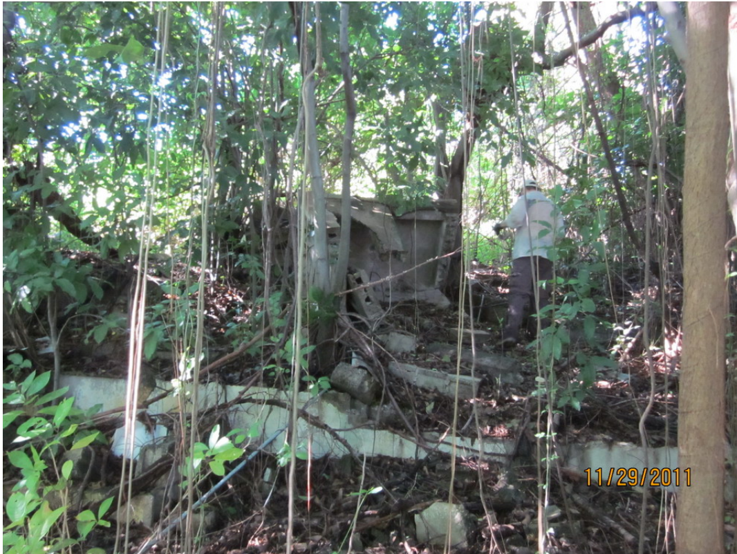
Figure 6. Typical view of the concrete and metal debris on the ground surface at Ponce Mameyes tower site
