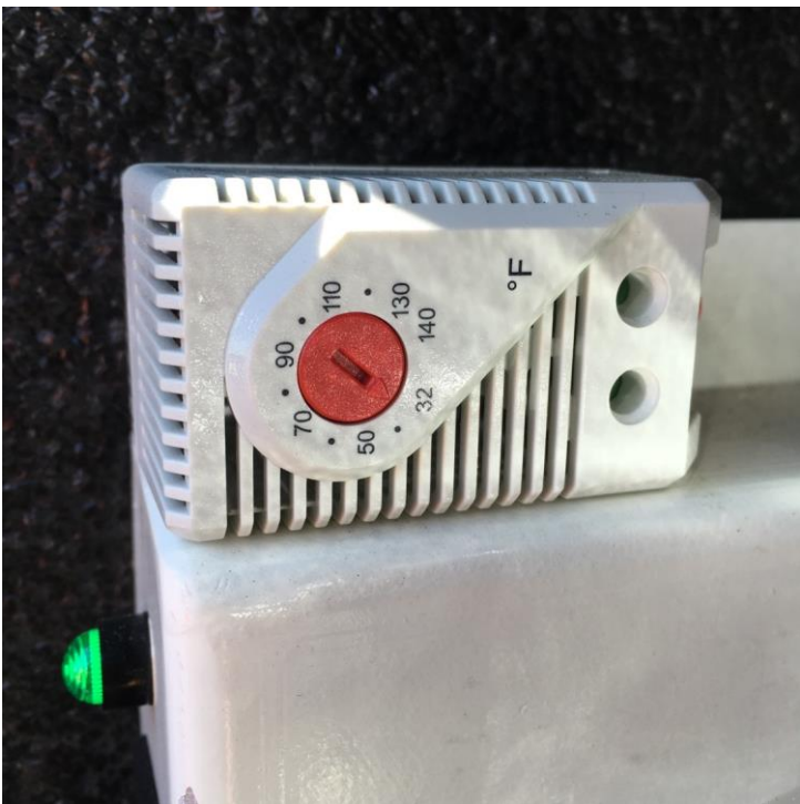
Figure 8. A view of one of the internal Temperature Controllers. See Figure 5 for the location of this Temperature Controller.
