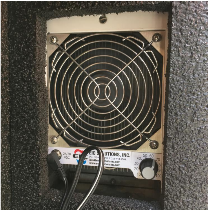
Figure 9. View of the Thermo-electric chiller unit from inside the enclosure (see Figure 5j for its location).
