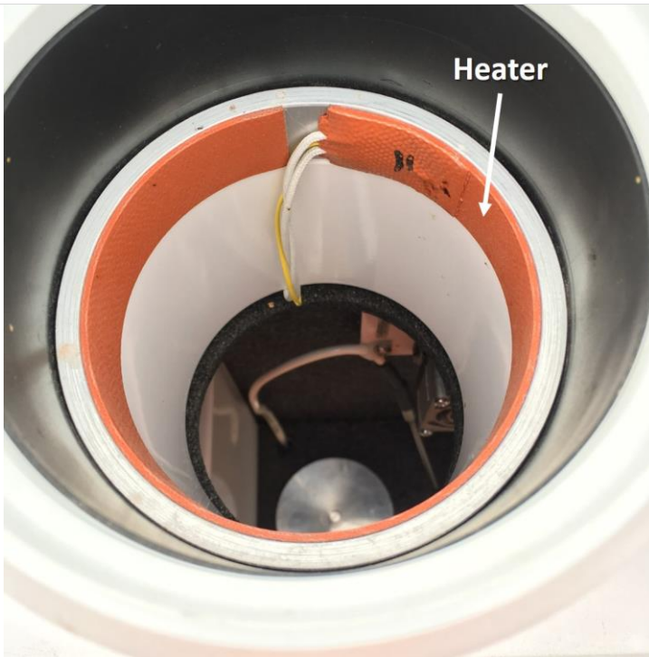
Figure 8. Inside each chimney is an automated silicon strip heater. This heater melts snow accumulation within the glass funnel.
