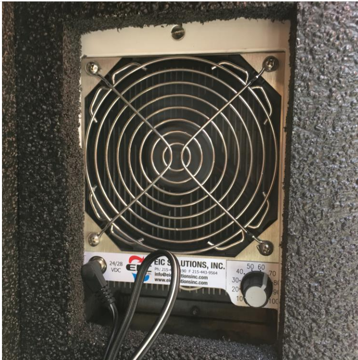
Figure 10. View of the Thermo-electric chiller unit from inside the enclosure (see Figure 5 for its location).
